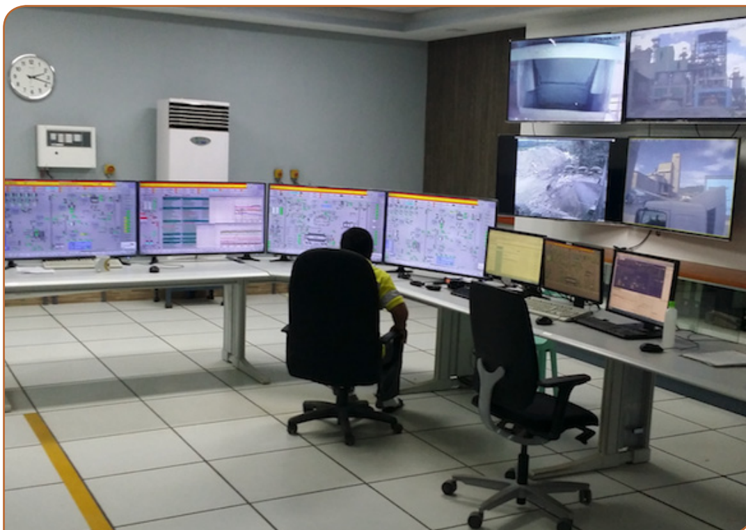
Left: Central control room at the Teresa plant, following the upgrade.
