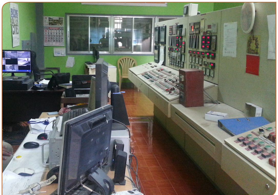
Right: Central control room at the Batangas plant, prior to the upgrade.
